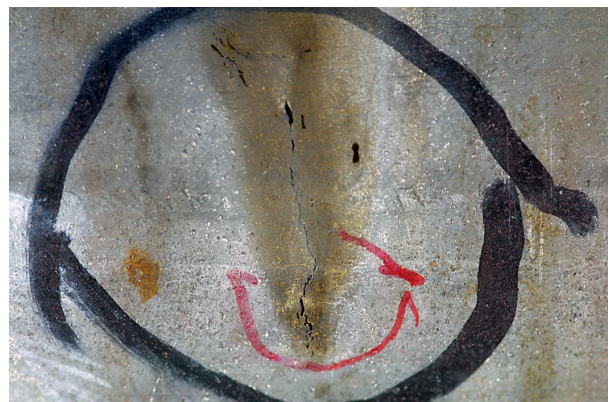
Fig. 4: Detail from image 3: place of damage with crack field \approx 3:1
